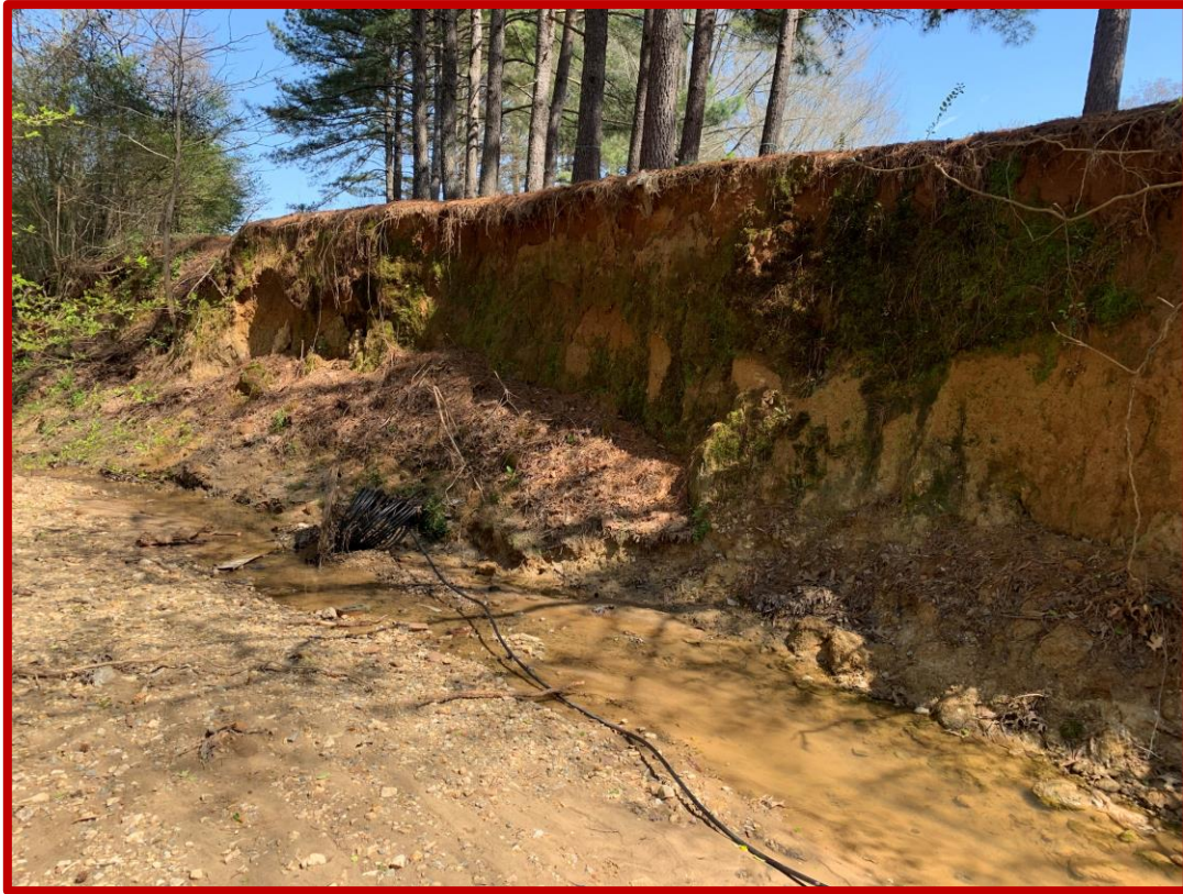
Photo 9: Representative Streambank Erosion
