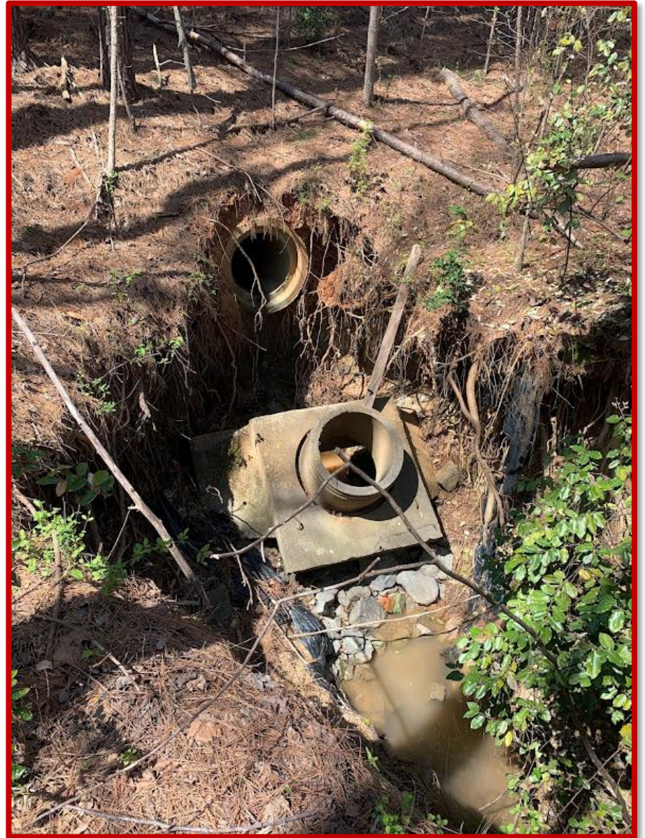
Photo 12: Representative Streambank Erosion
